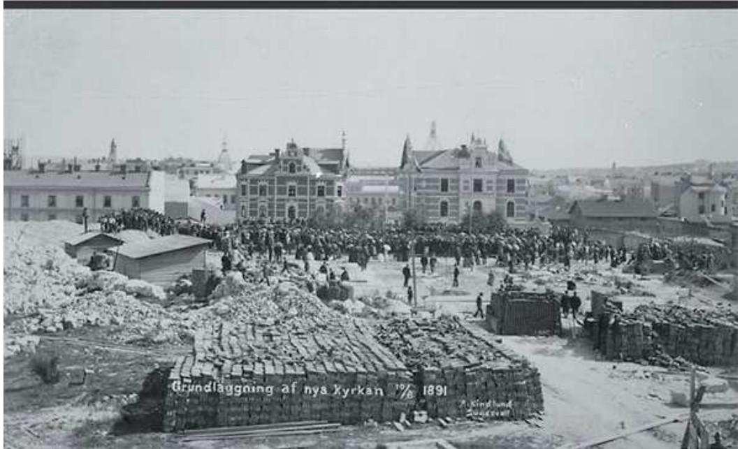
Photograph of the foundation of Sundsvall's new church 1891st Photo: Adele Kindlund.
